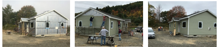
St. Mary's Catholic Church sent their "siding crew" to Lot #2 and finished in one day!
