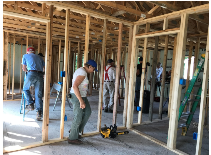
Volunteers working on framing out interior walls inside house #4 at McFarland Meadows.
