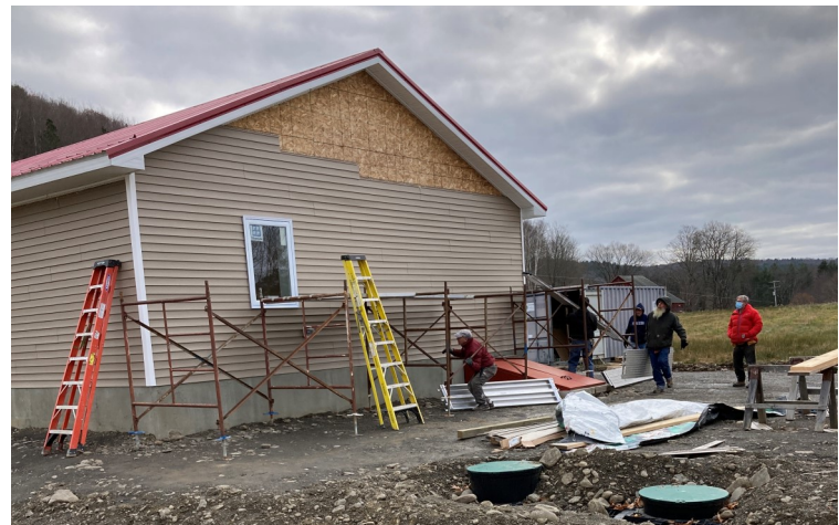
The last of the siding going up on lot #4 at McFarland Meadows just before we finished work in fall 2021.
