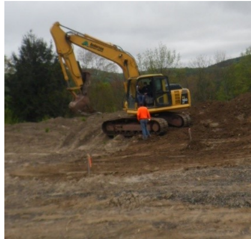
Parker Excavating working on the foundation of the first building site at McFarland Meadows.
